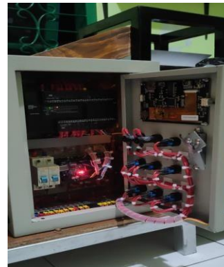
Gambar 4.3 Box control panel
